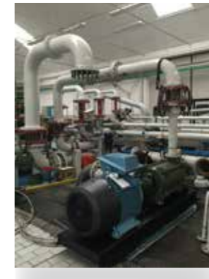
Figure 14 - Individual Pump being tested
