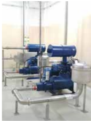
Figure 3 - Rotary Blower Installation in Food Industry
